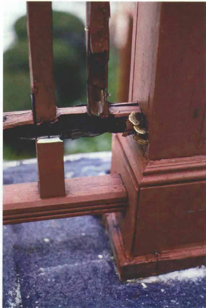
Mushrooming problems. When fungi sprout from railings, it's a rotten sign. Pictured here is a close-up of the railing the author was hired to replace.
